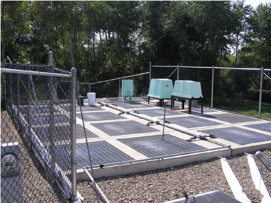
CUSTOM 40,000 GPD COMMERCIAL PLANT
